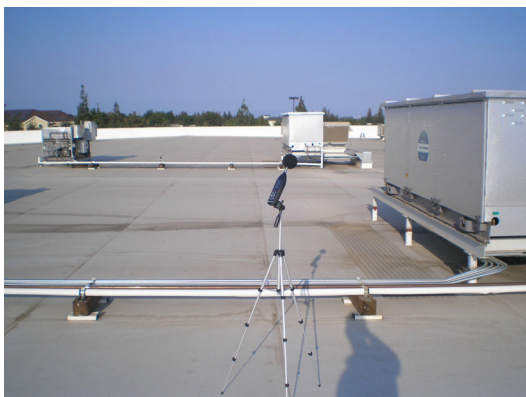
Rooftop Mechanical Equipment Noise Measurement
