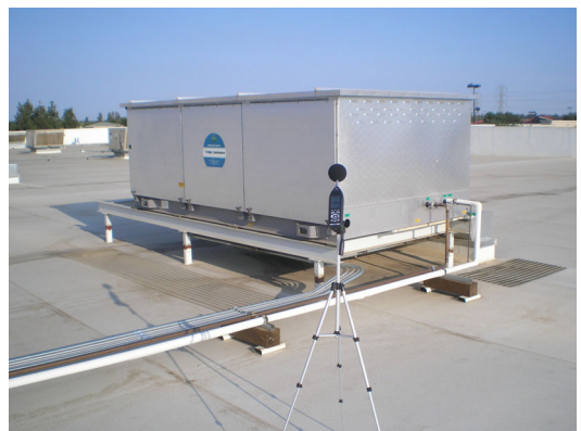
Rooftop Mechanical Equipment Noise Measurement
